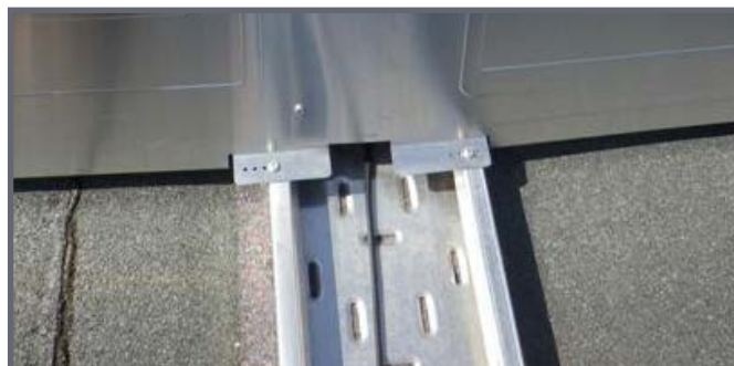
Wind deflectors fixed to floor rail
